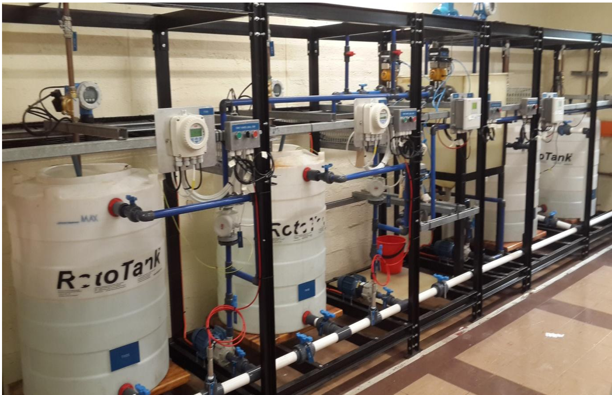
Figure 5.1: pH neutralization pilot plant used in real time experimentation.
