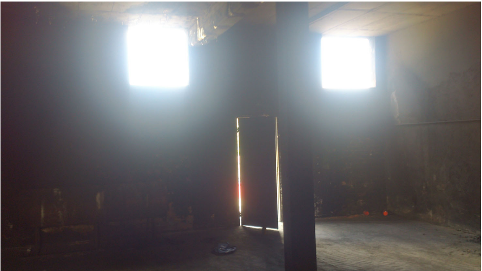
Figure 3. Inside the live fire training structure, facing the rear of the structure.
