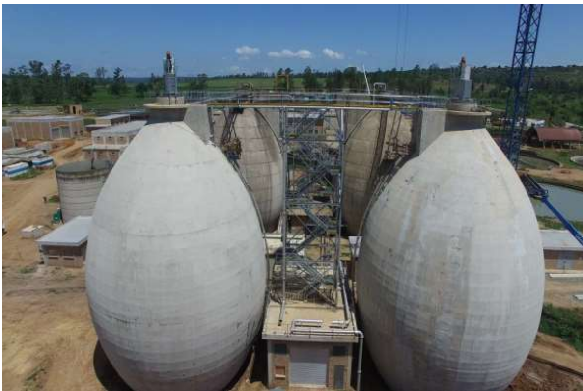
Figure 1.1 Egg-shaped anaerobic digesters used in the treatment of sludge obtained from Darvill Wastewater Treatment Plant
