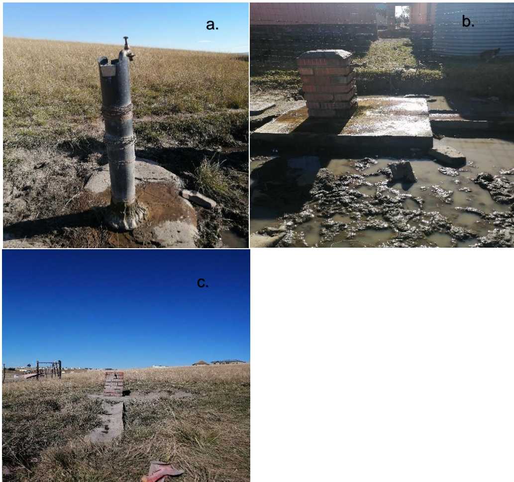
Figure 3-3: a. Yard tap, b. Leaking communal tap, c. Estranged communal tap
