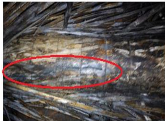
Figure 10. Mechanical cracks in varistor elements.
