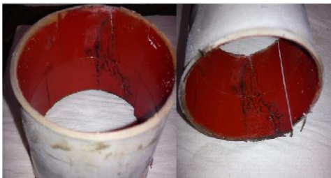
Figure 15. Treeing inside the sealing collar.
