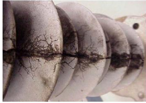
Figure 9. Deterioration on insulation housing [17].
