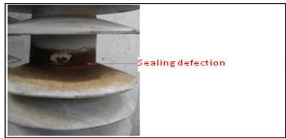
Figure 5. Sealing collar defective [14].
