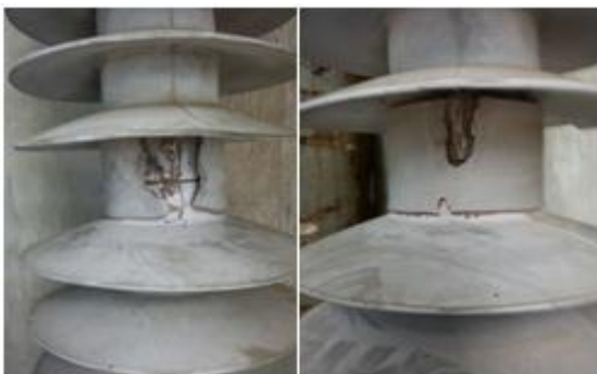
Figure 8. Defective sealing increase high rate of moisture ingress.
