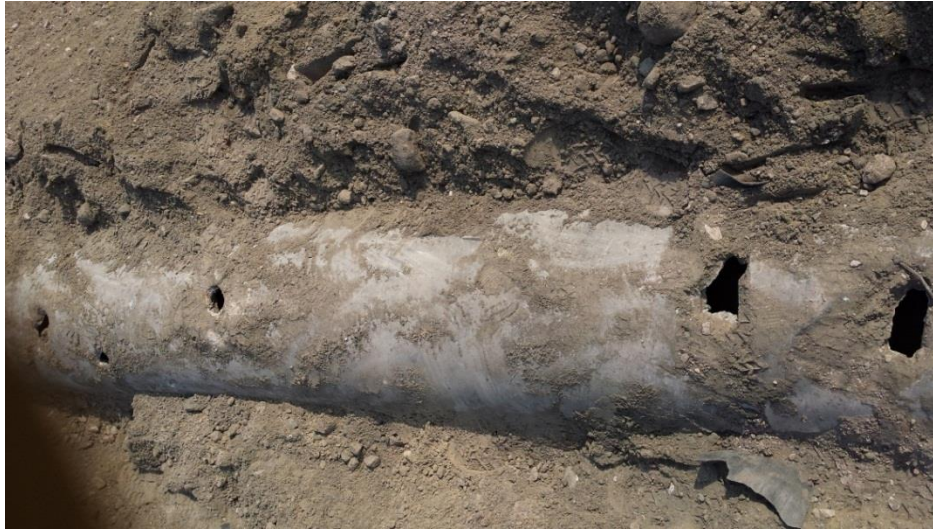
Figure 9: damaged stormwater pipe
