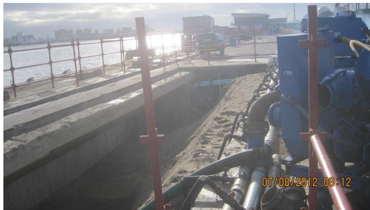
Figure 19: water pumps used
