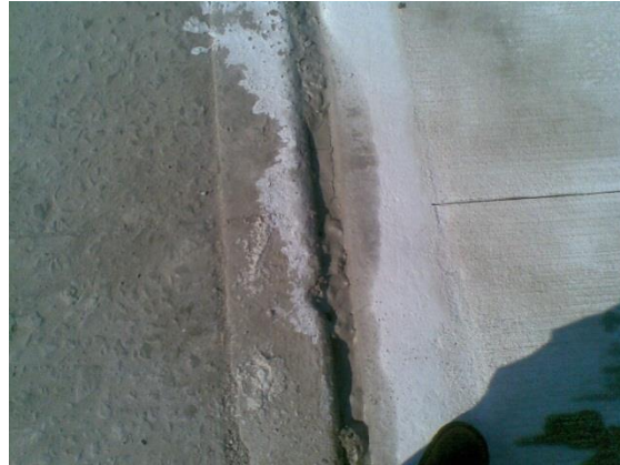
Figure 12: blocked slot drain
