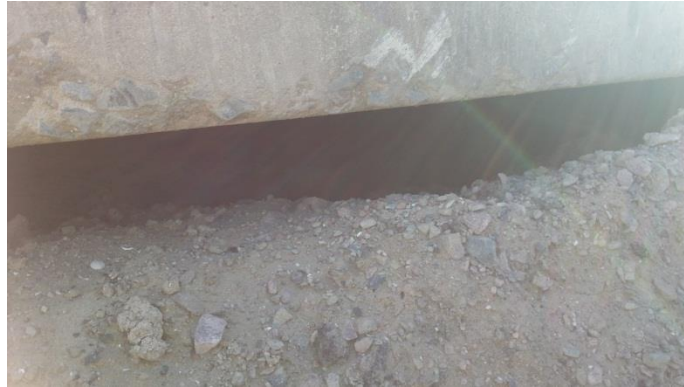
Figure 18: destabilization of the layerworks
