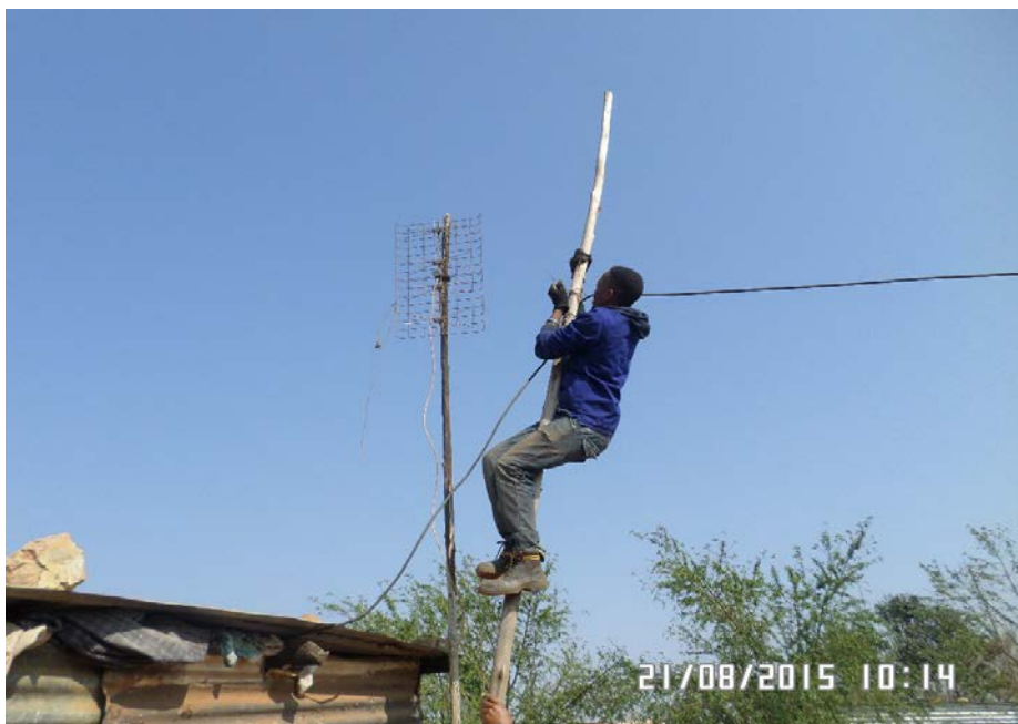
Figure 4: Gauteng informal settlement: dangerous and illegal connection of electrical cable to a facility
