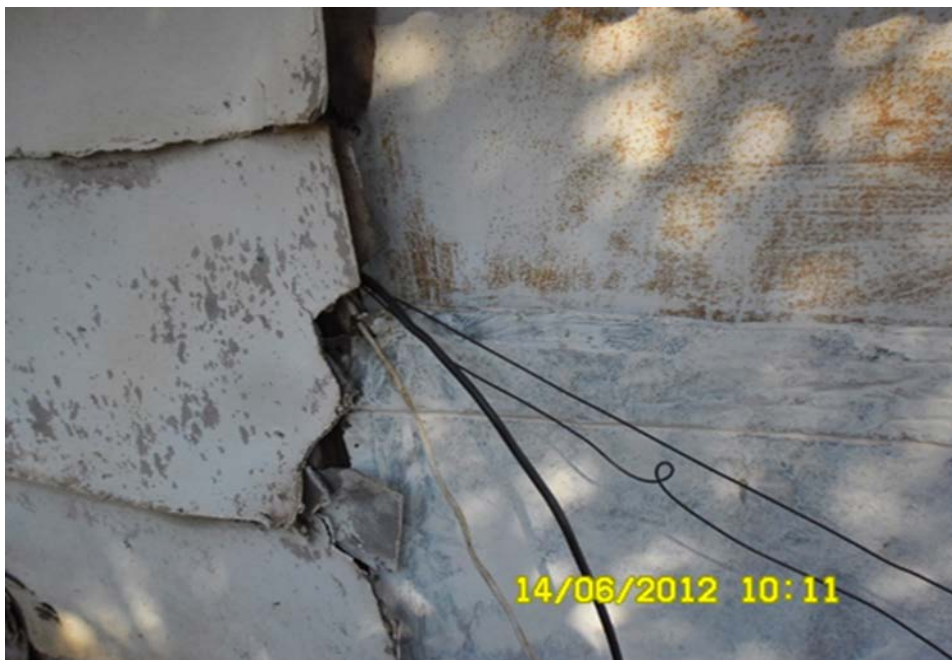
Figure 2: Illegal connections at Gauteng, Pretoria
