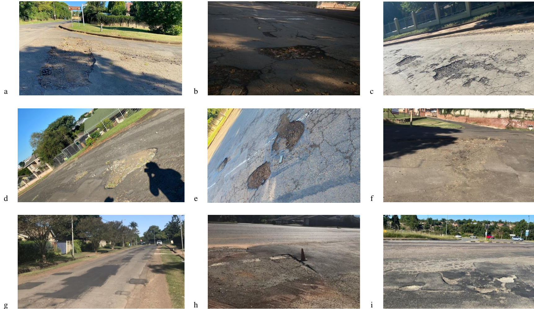
Figure 9: Road riddled with potholes (a - f) and the good to poorly repaired roads (g - i)
